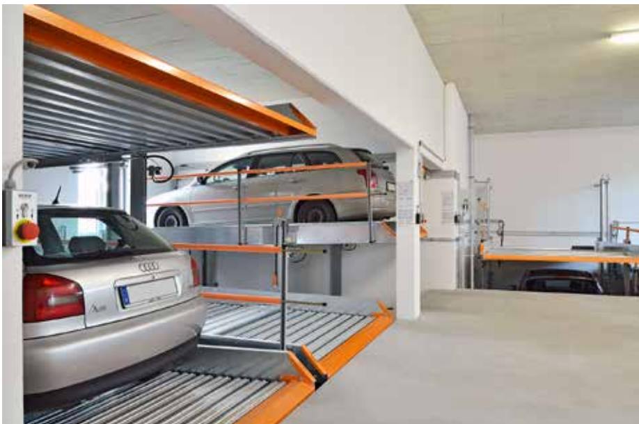
If your apartment block uses car stackers, you may not always get the same parking bay, making EV charging more complex. Image: KLAUS Multiparking ANZ
