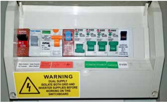
← This switchboard has two spare slots (at right)—plenty of room to add another EVSE (if the supply is available!).
